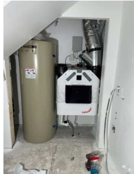
The heat recovery ventilator and hot water storage tank being installed in a crawl space under the stairs.
