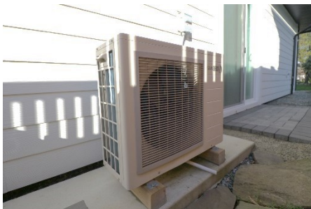
This one heat pump outdoor unit provides enough energy for both space heating and hot water.
